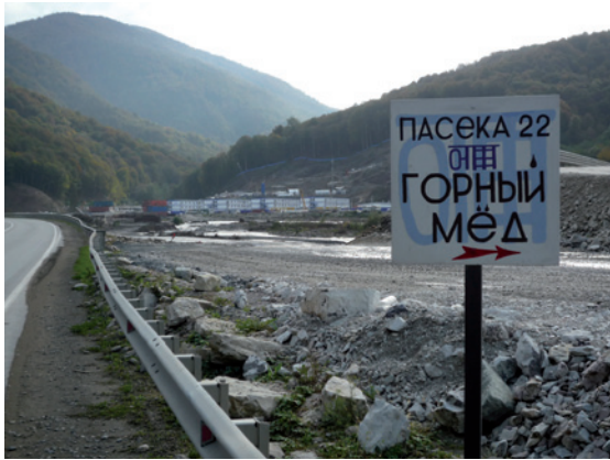
Figure 7 – From Adler to Krasnaia Poliana and far into the Mzymta valley, for more than 50 km one building site borders on the next. Here they are constructing the second road on the left bank and a railway line along the Mzymta. The sign pointing to beekeeping station no. 22 and the sale of mountain honey seems almost surreal given the dust-laden reality. © K. Scharr 2010
