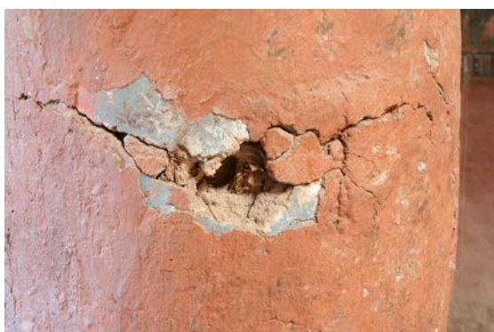
Fig. 3.5 (Left) Basgo. Maitreya Lhakhang. Fibres visible due to a damage of the plaster.
