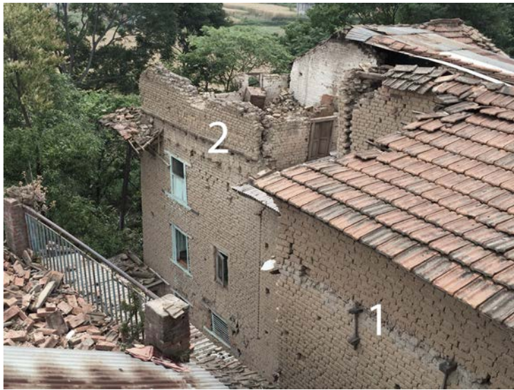
Fig. 4.15 Kathmandu Valley. Nepal. 1 = Wooden wedges as a traditional technique to stabilise walls. 2 = Wooden components destroyed during the earthquake in 2015. Photo: Christof Ziegert.
