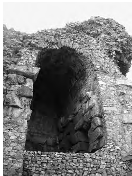
46 Northern substructure chamber with a deep crack running along the vault and back wall
