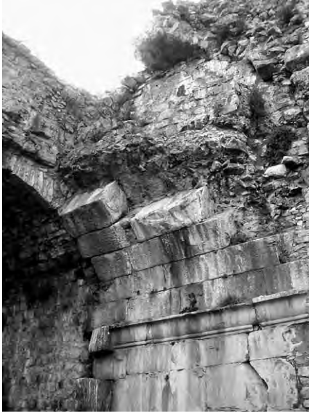
42 Marble vault blocks in the south analemma in danger of collapse
