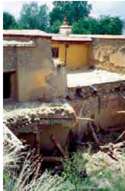
23–24. Lessons in Impermanence: Remains of the Western and Eastern Glo-'bur (2001)
